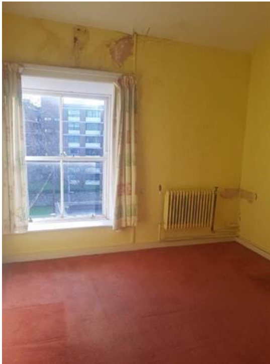
Plate 158: 2 nd floor level typical study room to front (east) on first floor with signs of water damage
