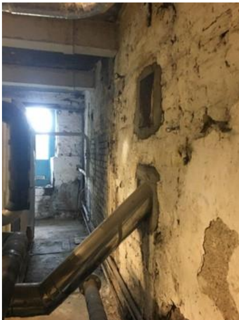
Plate 104: Former kitchen to northwest at basement level, with original masonry and floor flags evident. Note concrete downstands for concrete floor plate supporting entrance level above
