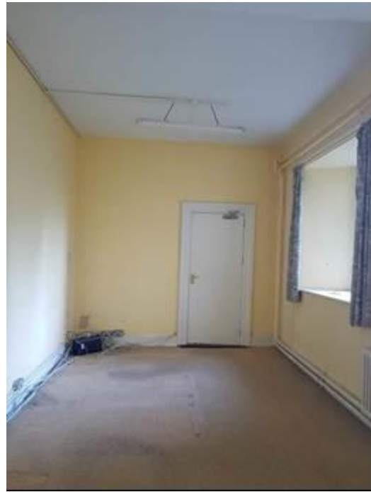
Plate 233: A typical dormitory showing signs of water ingress beneath floors
