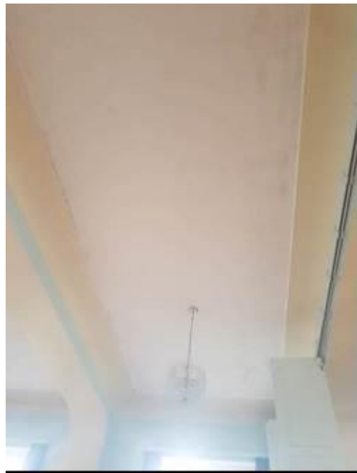
Plate 250: Ceiling showing some signs of water damage
