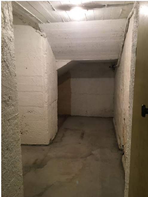
Plate 100: Early masonry with concrete supports to concrete stairwell, note concrete ceiling slabs above
