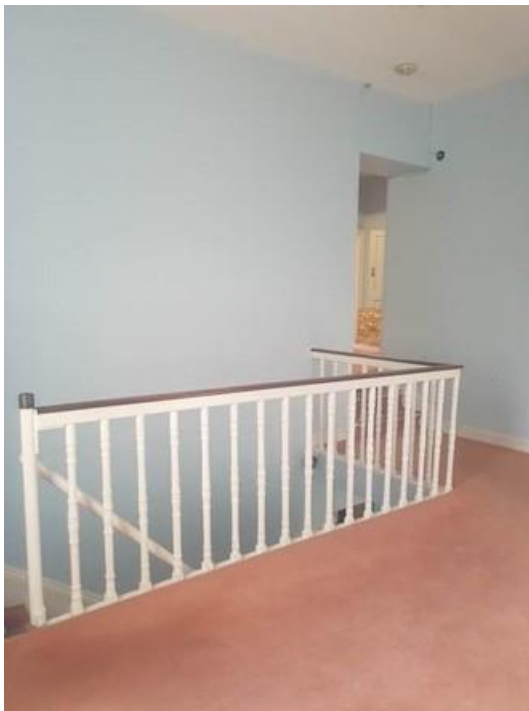
Plate 114: Landing with mahogany painted stair rail leading to 1 st floor level below
