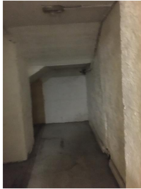
Plate 99: Void under concrete stair
