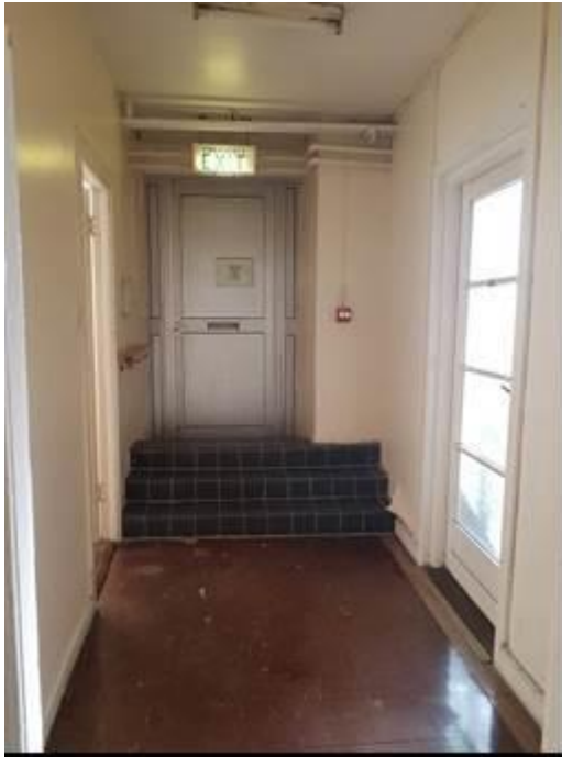
Plate 255: Fire door within central corridor with flood relief barrier evident
