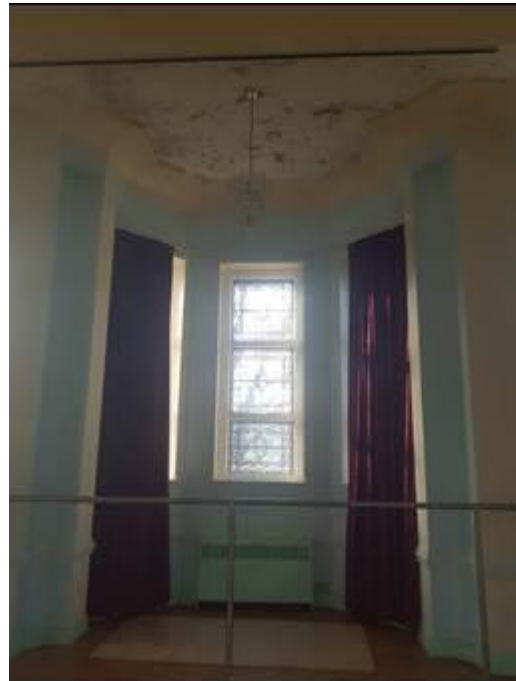
Plate 246: Leaded windows in apsed southern gable. Note water ingress at ceiling level
