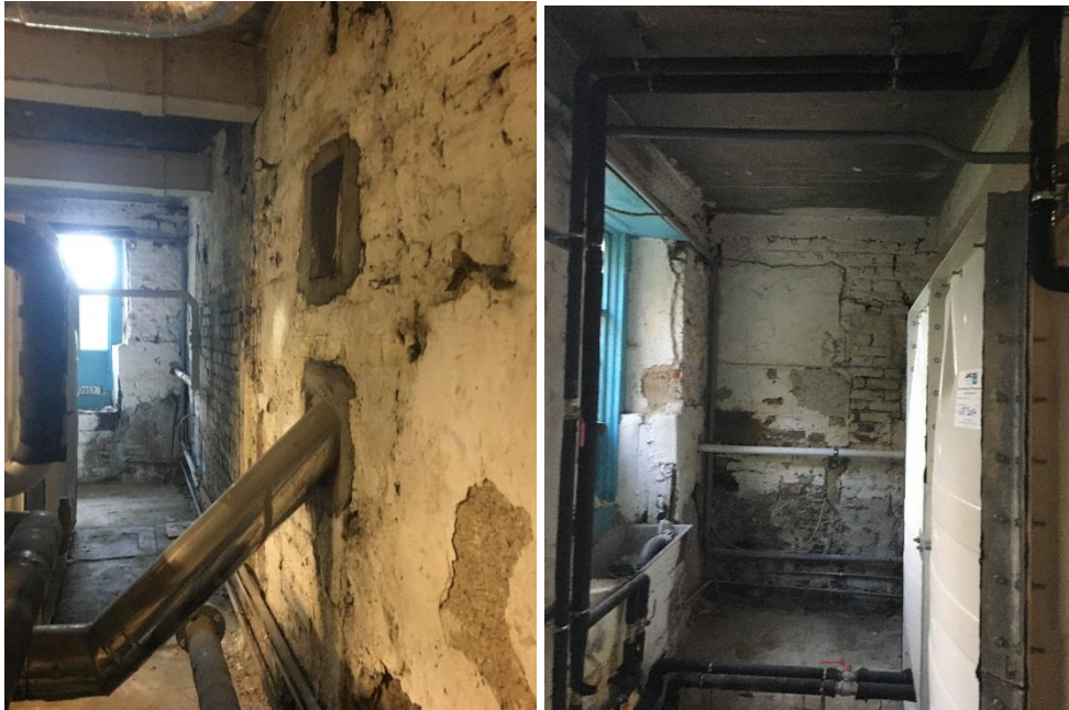
Fig.29 Former kitchen to northwest at basement level, with original masonry and floor flags evident. Note concrete downstands for concrete floor plate supporting entrance level above. Fig.30 View east in same room
