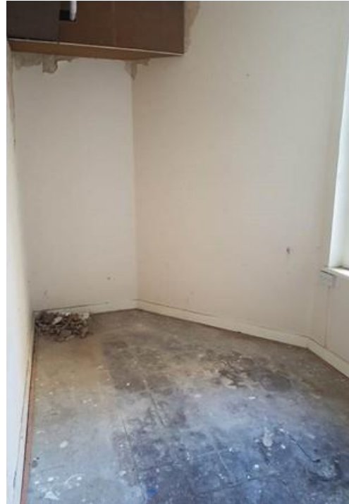
Plate 134: Small room with partitioned wall showing signs of water damage
