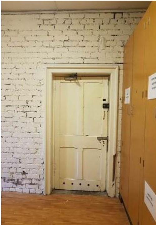
Plate 186: Services area at lower ground floor level with original walls exposed and painted
