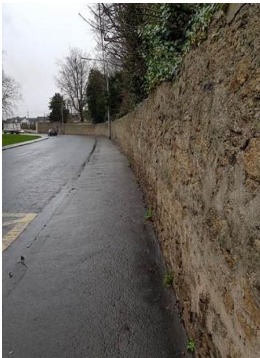
Plate 75: Curve of wall looking up Milltown Road towards new entrance, note multiple pointing types cement repairs to rubble wall
