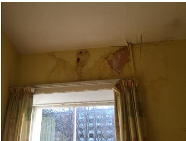
Fig.31 Example of decay due to water ingress from breaches in roof coverings, at 2 nd floor (later intervention) level
