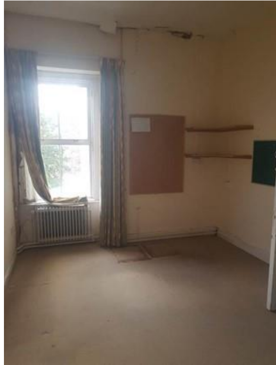
Plate 121: Sample room within vertical extension above main house. Note water ingress from breaches at roof level
