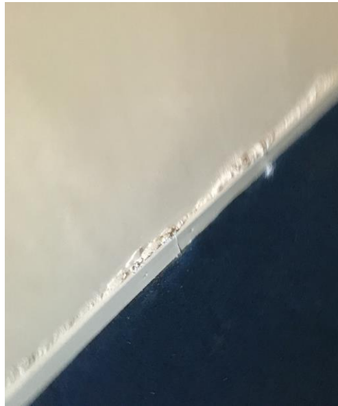
Plate 103: decay of skirting boards within corridor
