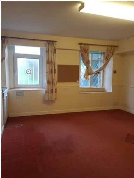
Plate 129: Dormitory at lower ground floor level. Note water ingress
