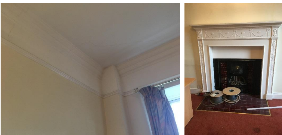
Fig.27 Overpainted stucco cornice, with services riser in corner.
